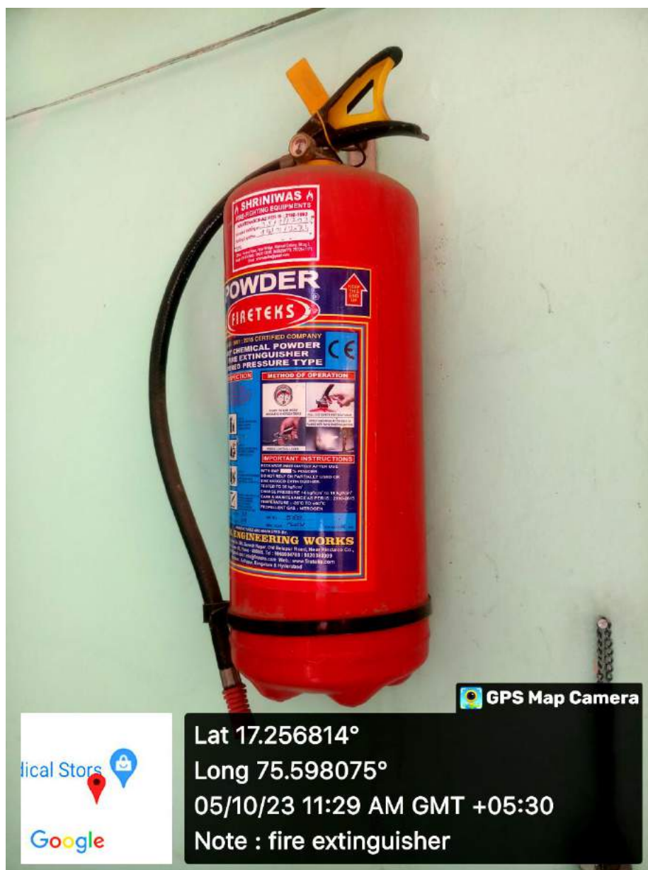
Fire Extinguisher in Laboratory
